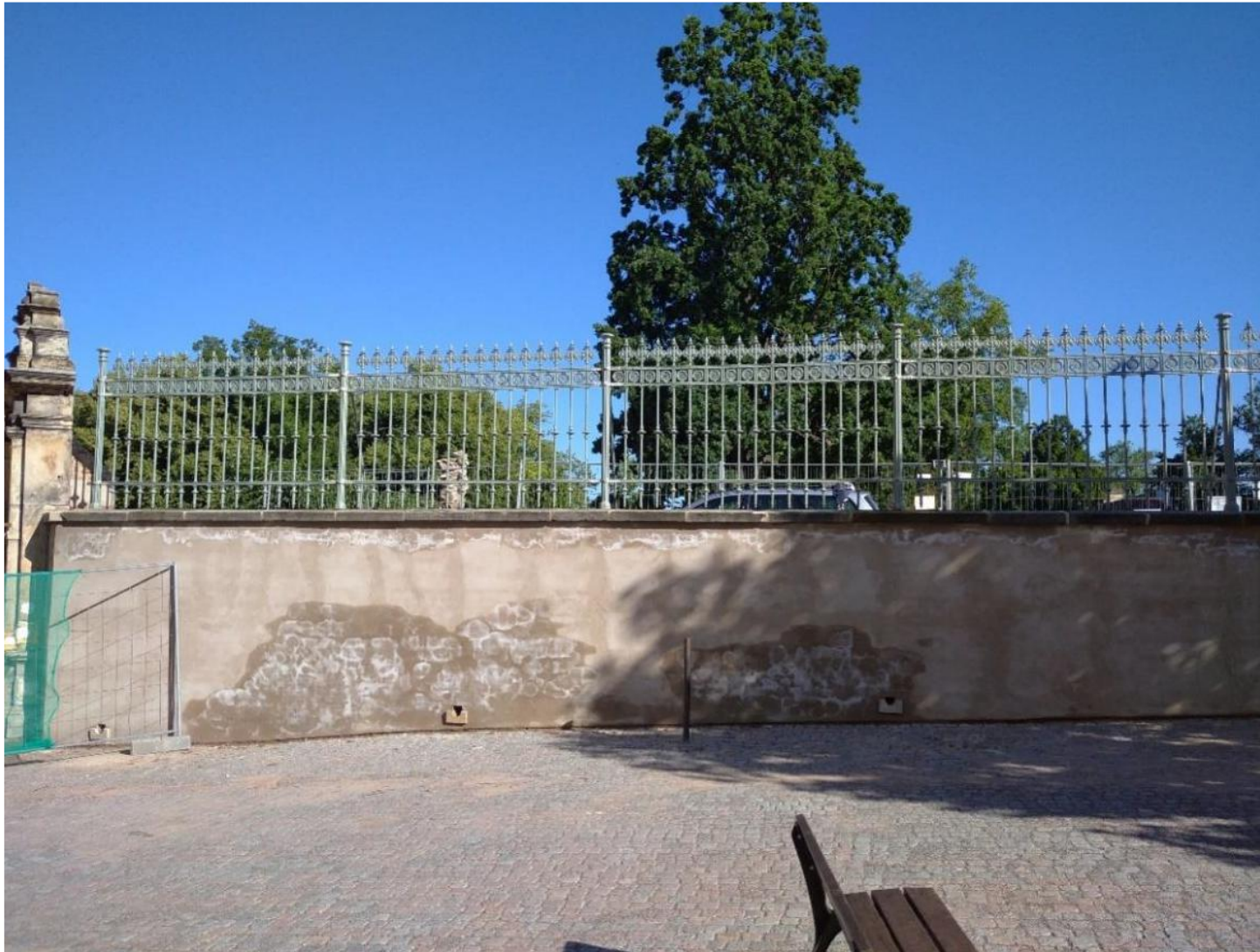
Damage several months after completion
