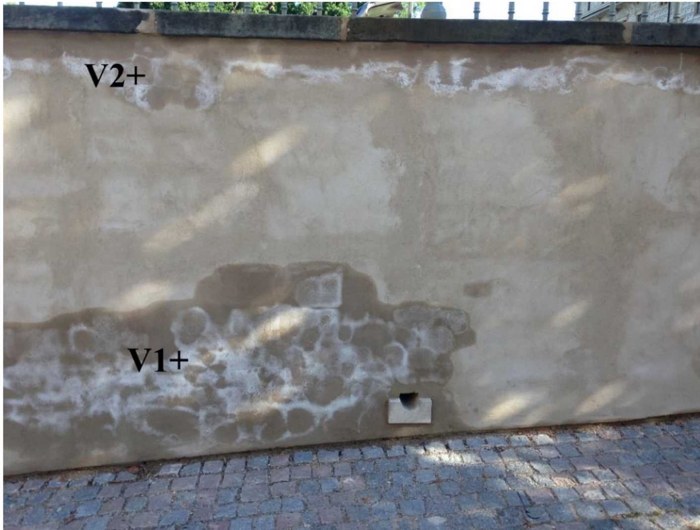
Damage several months after completion
